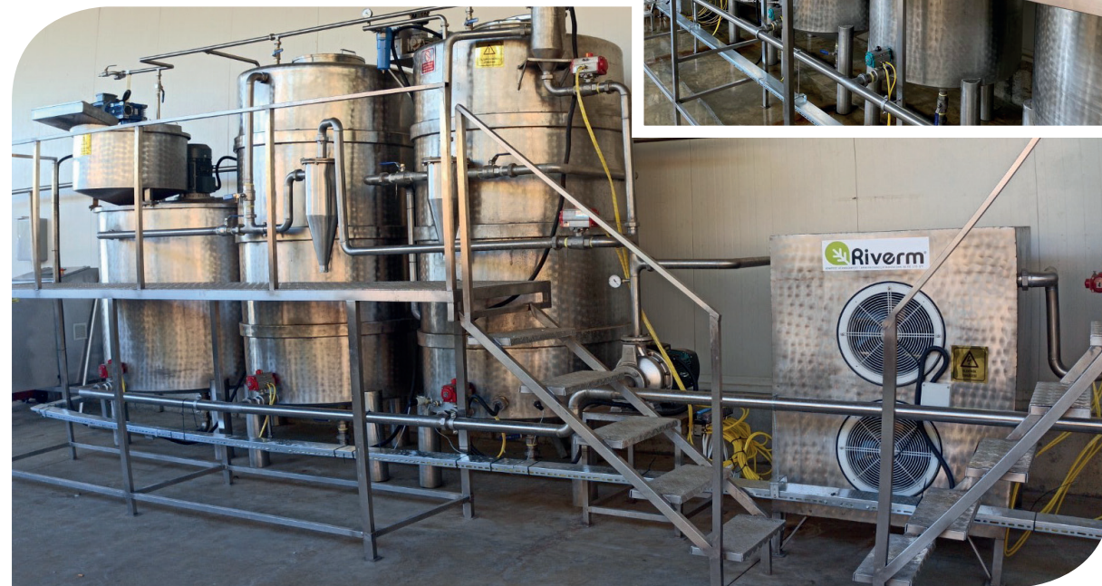
Production capacity 2 tons.
